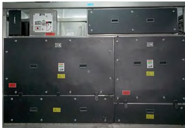
Outside view of traction converter
