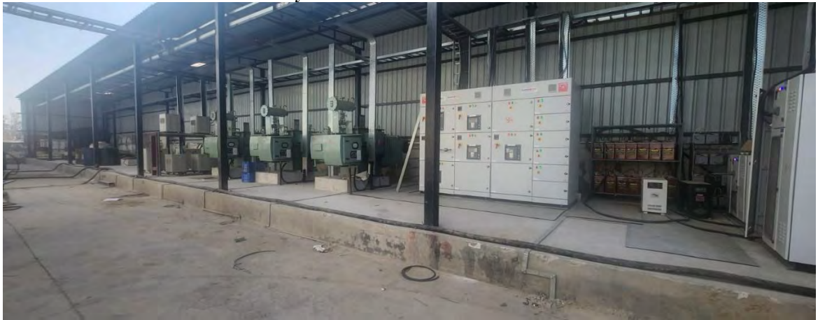
Transformers for Test Set up
